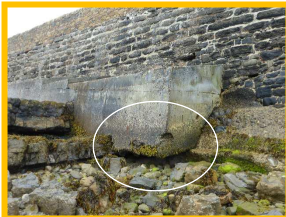
Undermining of seawall at Beadnell North (Nacker's Hole) (/1701C36)
