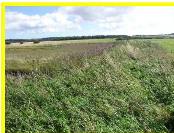
1401C21 – Heavily overgrown embankment to rear of saltmarsh
