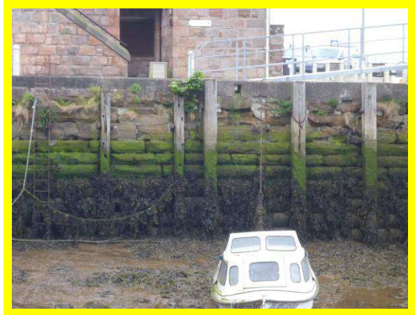
Masonry quay walls in dock area in fair overall condition with some open joints, cracks and abrasion (/0801C03)
