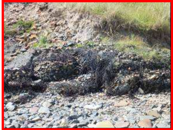
Failed section of gabion (/3201C22)
