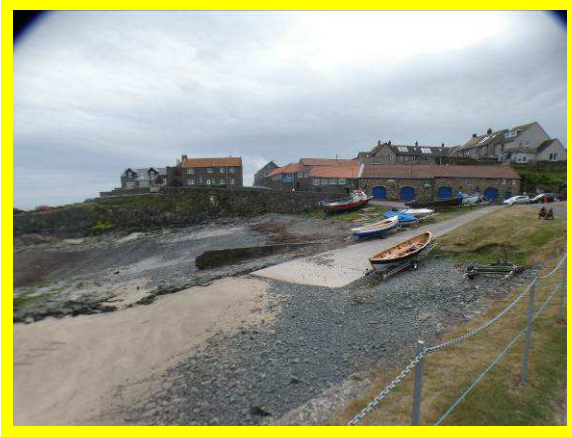
Slipway with slight voiding at toe (/2201/C06)
