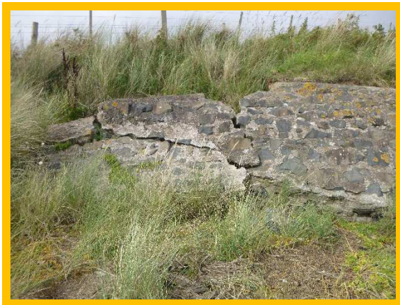
1401C29 – Extensive damage to western end of revetment.
