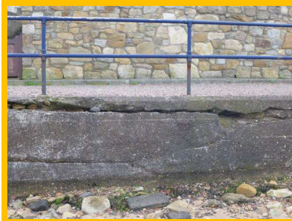
Sea wall along Bay View in poor overall condition (/3001C10)
