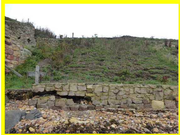
Damage to retaining wall adjacent lime kiln. Possible slumping of slope to rear (/1701C44)
