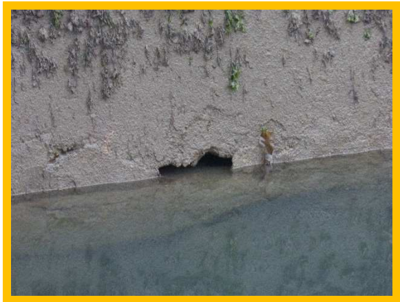
Scour hole visible along inner face 1701/C14
