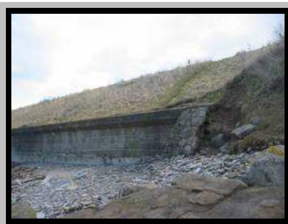
Outflanking of northern end of wall 1701/C54 - 2006
