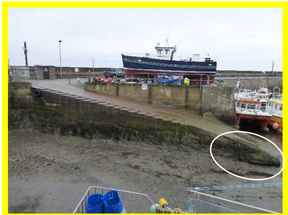
Undercutting of slipway 1701/C12
