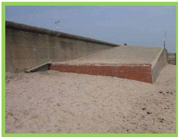
Low beach levels at ramp new end of promenade (4201C07)
