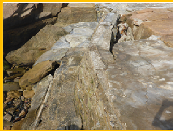
Voiding at crest of small wall
