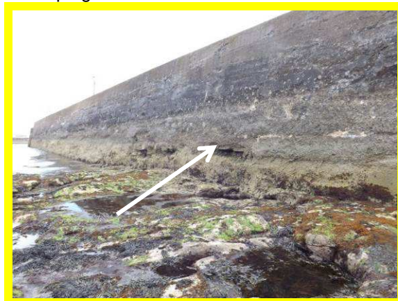
Increased depth of abrasion hole 1701/C07 2016
