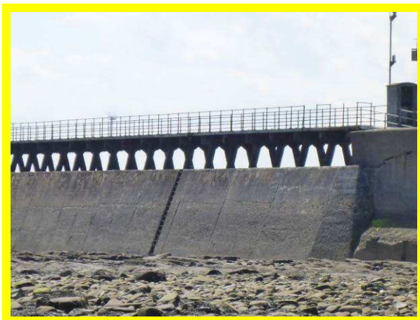
Generally fair condition of main Blyth East Pier substructure (although superstructure in poorer condition) (4001C05)
