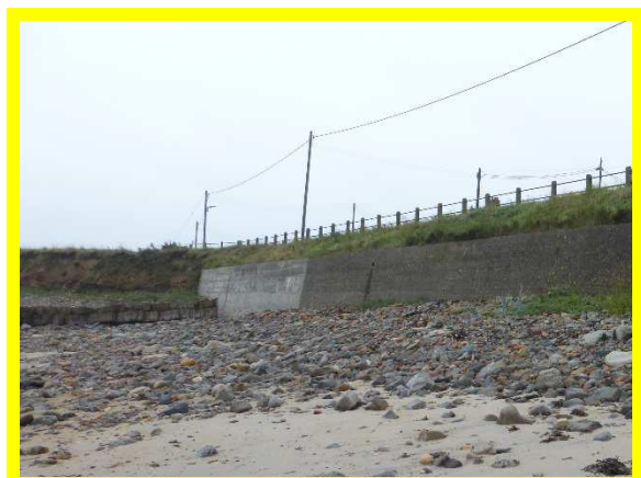
Fair classification of wall north of Dell Point, minor outflanking at southern end (/1701C27)
