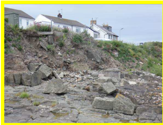
Slight erosion around outfall (/2201C02)
