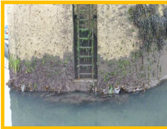
Possible signs of undermining around nose 1701/C14
