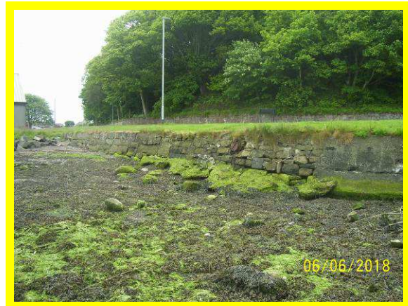
901c05/06 in 2018 showing some possible erosion but little overall change from 2008.
