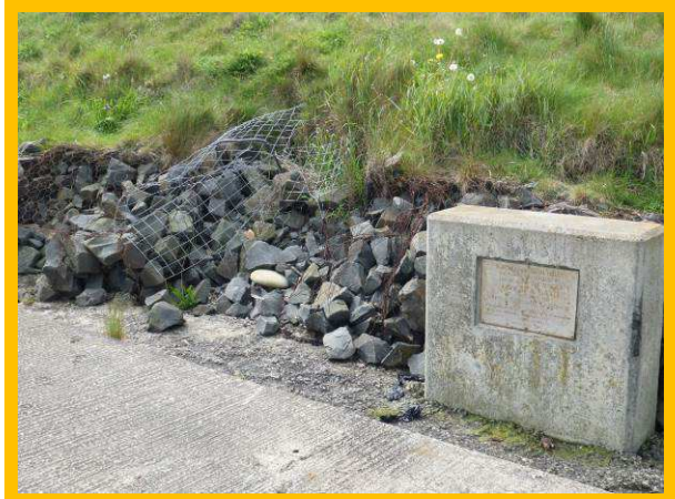
Break-up of gabion baskets (/4401C19)
