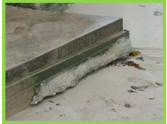
1701/C16 Low beach levels have exposed toe of steps, wall remains in good condition,
