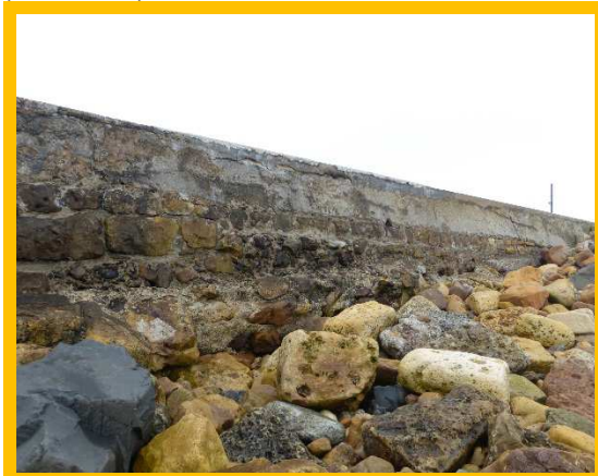
Abrasion and undermining of Beadnell Harbour wall (outer face of eastern wall) (1701C47)
