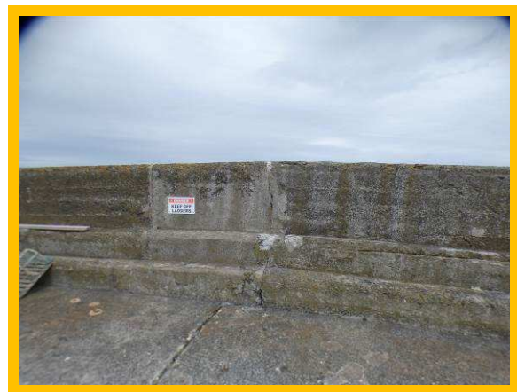
Inside face (crest wall) at crack (/2201C03)
