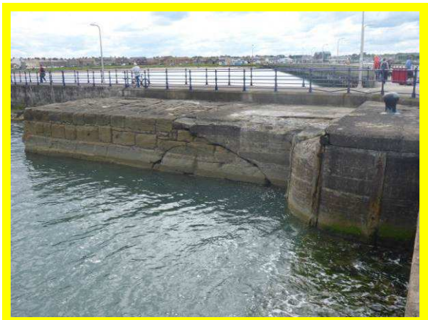
Poor condition at junction of South Pier and South Jetty (seaward face) (/3101C01)
