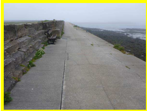
Older (inland) sections of cracked deck and abraded wave wall on Berwick Pier (/0701C14)
