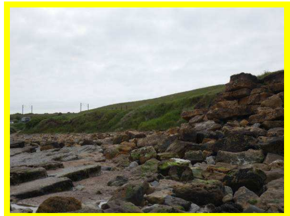
1101/c05 Critical section of frontage closest to road 2018.
