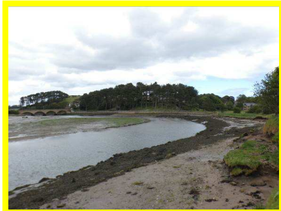
Eroding face of raised area (/2801C09)
