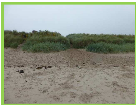
1701/C23 localised evidence of erosion at beach access points.
