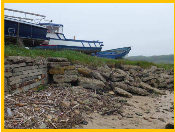
Failed section of Wansbeck Boat Club retaining wall (/3801C02)
