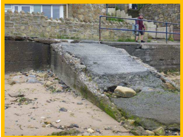
Access ramp to Little Shore Wave Basin in poor condition (/3001C10)
