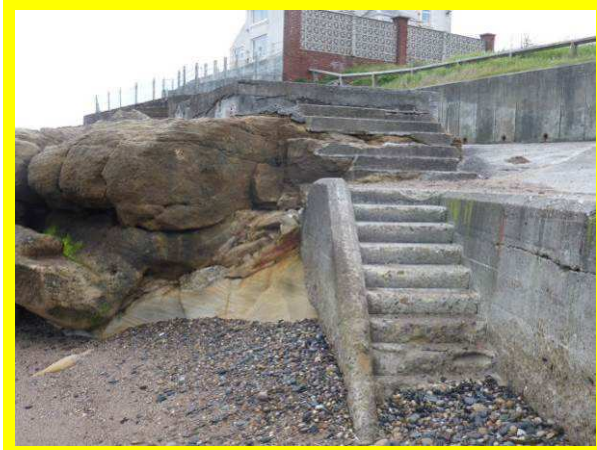
Heavily abraded access steps to foreshore (/3101C02)
