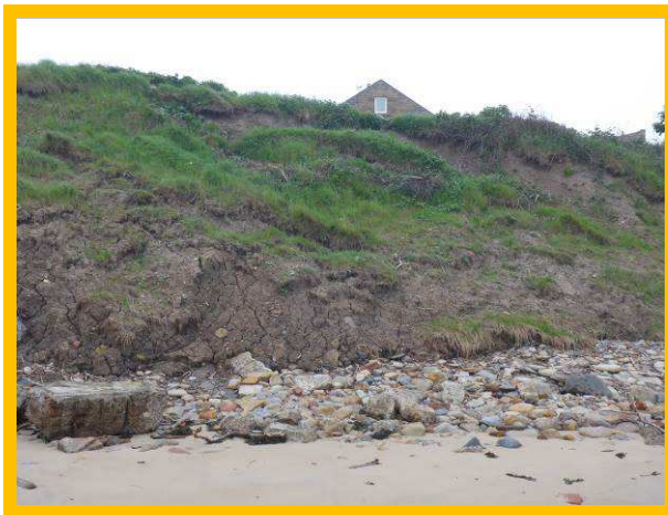
Eroding cliffs south of Cambois House (/3901C01)
