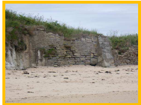
Poor condition retaining wall (/2501C01) 2018
