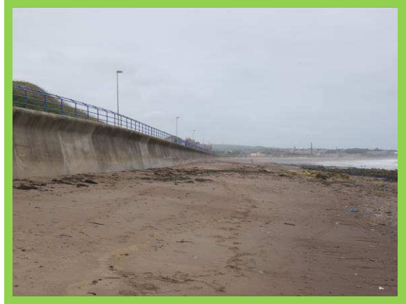
1001 c03 – slight reduction in beach levels at northern end 2018.
