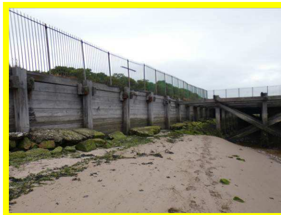
901c07 – reduced beach levels 2018, exposing support to structure.
