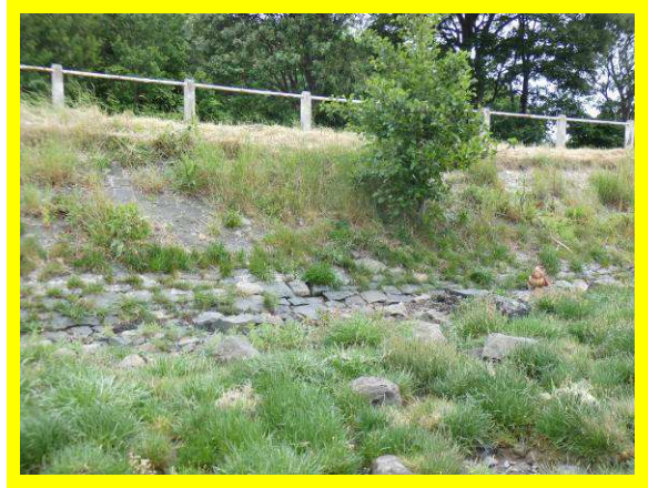
1501/C04 – gaps and local movement of stone to revetment.
