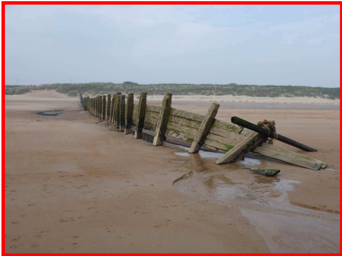
Failed seaward end of southern groyne (/4301C01)
