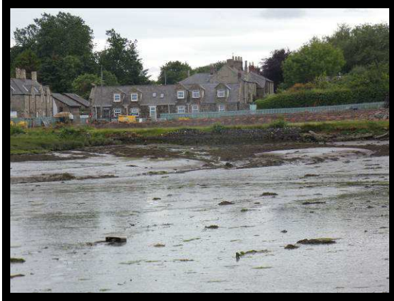
1501/C02 – poor condition of masonry wall but development occurring behind.
