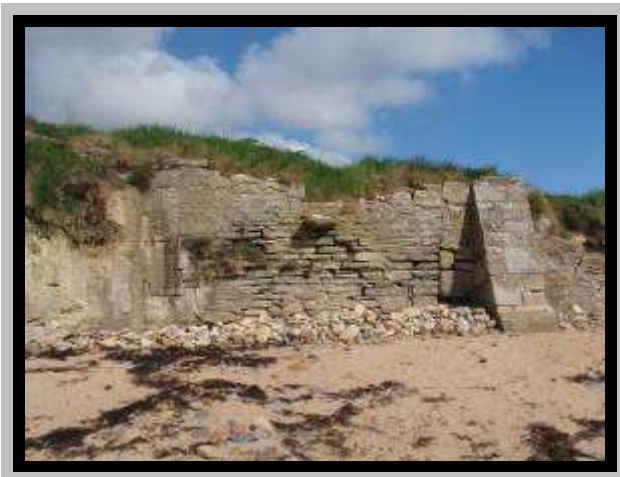
Poor condition retaining wall (/2501C01) 2016
