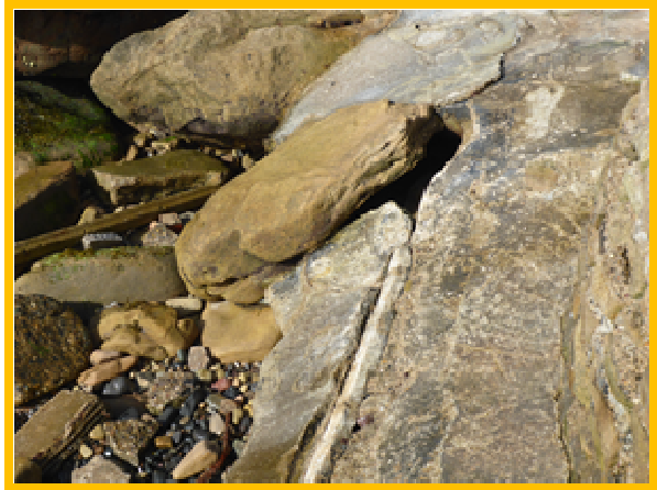
Undermining at toe of small wall
