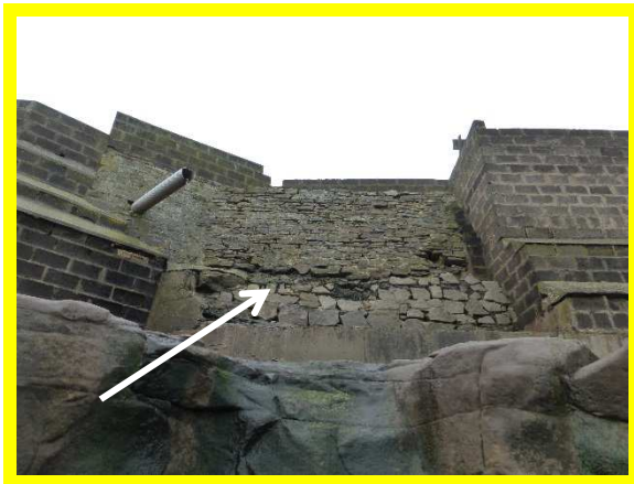
1701/C03, requires repointing.
