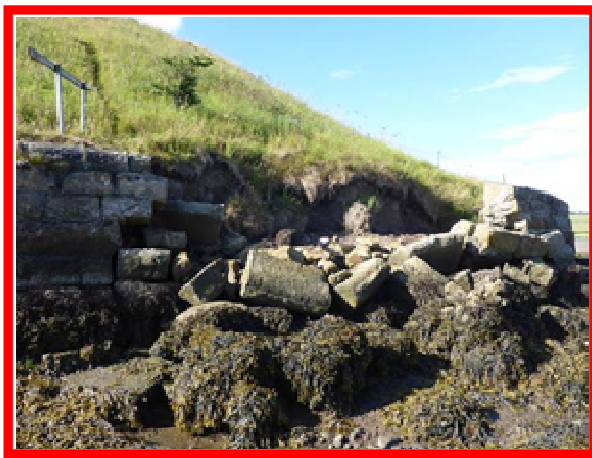
Collapsed section of wall at Church Hill now with erosion of the land behind (/2801C13)
