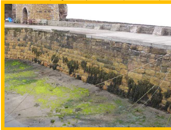
Open joints between blocks on Beadnell Harbour wall (inner face of eastern wall) (1701C51)
