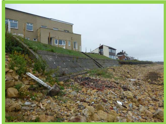
Concrete revetment in good condition, evidence of grout repairs at southern end (/1701C42)
