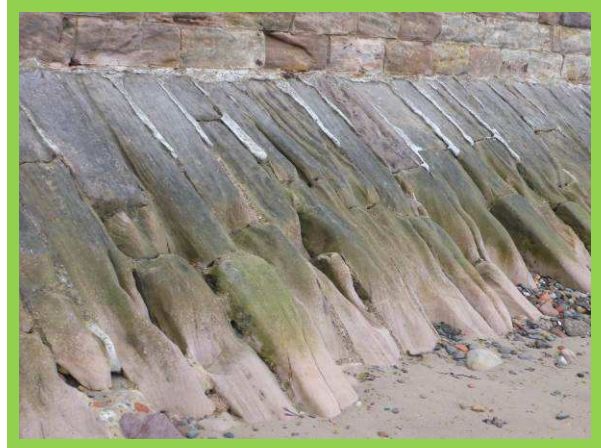
Abrasion to toe apron where present (/0801C06)
