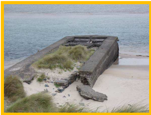
1501/C06 – Partial collapse of northern wall to jetty
