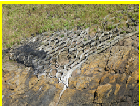
Hexagonal erosion control matting below castle in fair condition but locally with absent rocks (/4901c12).
