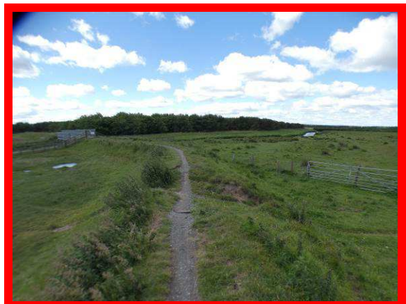
1401/ C31, Bank failure to area of South Low.
