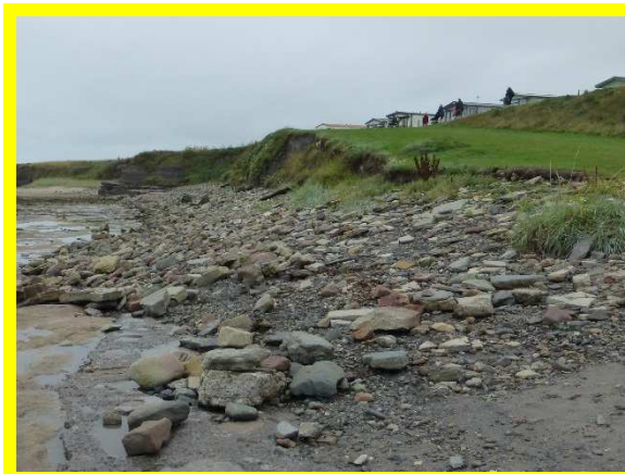
Erosion to access ramp 1701/ C22
