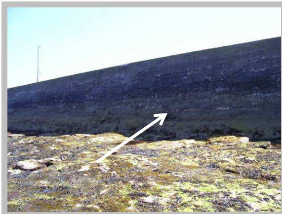
Developing abrasion hole 1701/C07 2010
