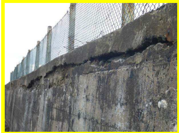
Cracks in private seawall around Pan Point (/3101C04)
