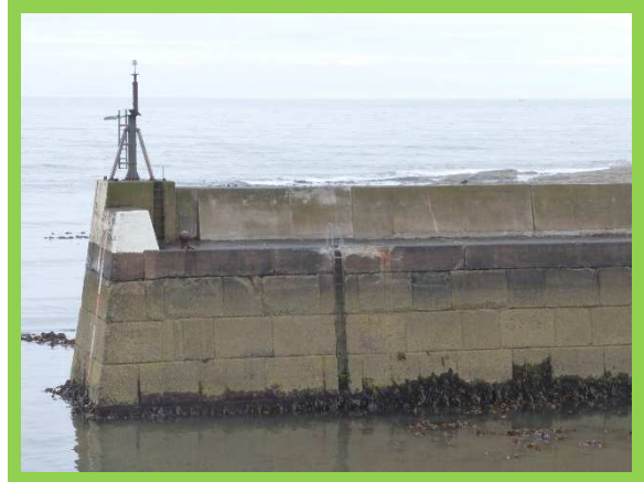
1701/C21 Good condition, some cracking and loss of mortar in original deck - no significant damage.
