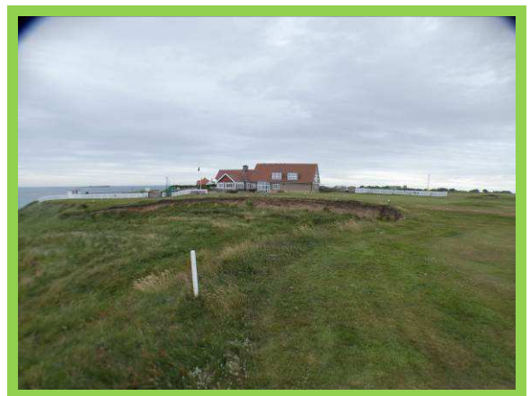
1501/C07 – slow continued slippage at crest of coastal slope.
