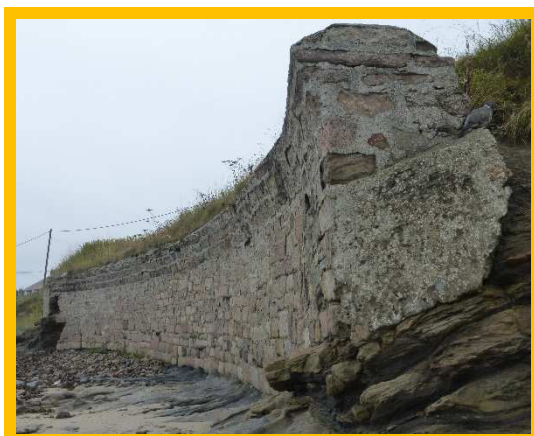
Masonry blockwork wall in poor condition. (/1701C25)
