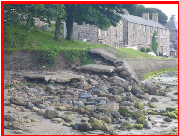
Local failed section of river slope revetment/wall (/0801C07)
