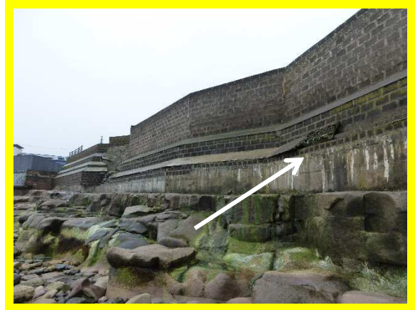
Damage of lower coping 2018 (1701/C02)
