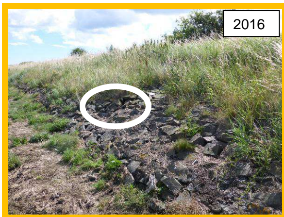
1401C98 – generally fair but locally poor stone-revetted embankment.
