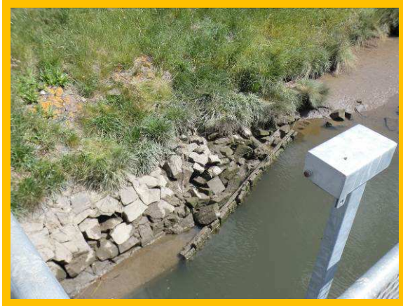
1401/C01 – undermining of edge protection.
