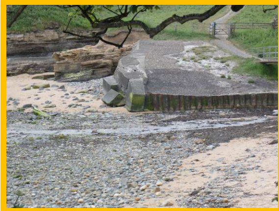
Undermining and voiding in concrete at southern bridge abutment (/2501C01). Low beach levels
