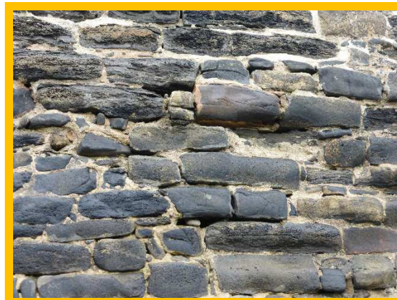
Loss of mortar and damage to blockwork of seawall at Beadnell North (Nacker's Hole) (/1701C36)
