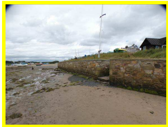
Masonry wall at Boat Club with some signs of loss of pointing. (/2801C03)
