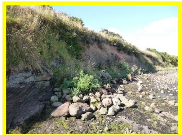
1401/ C23 Actively eroding sandstone escarpment along Common Slap
