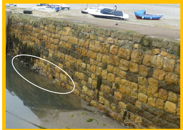
Undermining of Beadnell Harbour wall (inner face of northern wall) (/1701C52)
