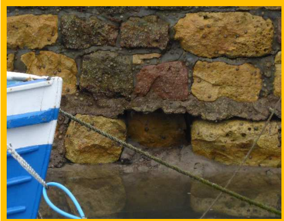
Missing block at toe of Beadnell Harbour wall (inner face of northern wall) (/1701C52)
