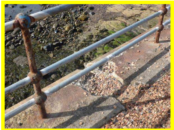
Local crest damage to Church Point seawall (/3601C12)
