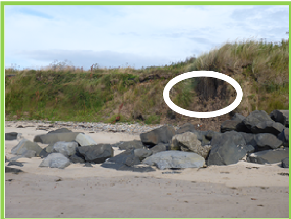
Erosion of low cliffs (/3201C14) at terminal end of rock revetment
