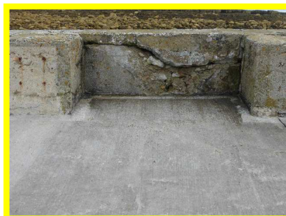
Damage to splash wall (1701C51)
