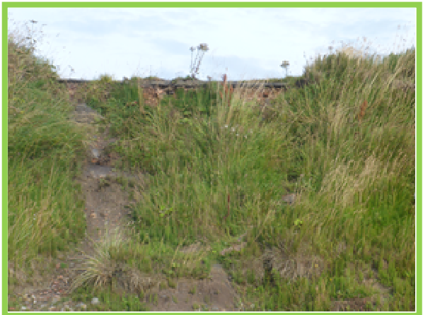
Erosion of low cliffs exposing carriageway of access road (/3201C14)
