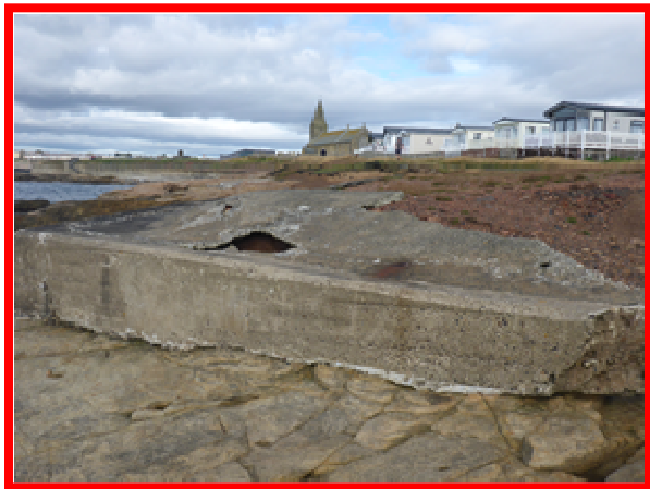
Seawall actively breaking-up since at least 2008 (/3501C10)
