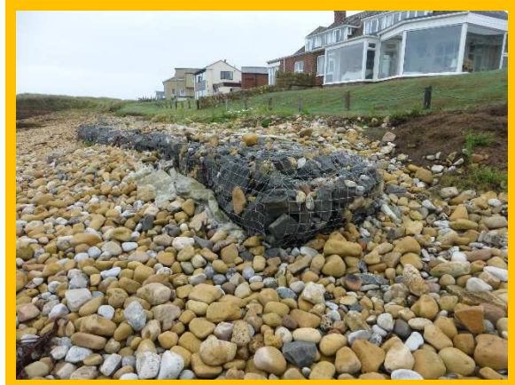
Damage to gabion basket wall at (Lady's Hole) gabion wall (/1701C40)
