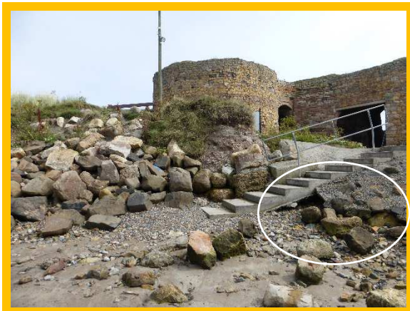
Undermining and partial collapse of grouted stone revetment adjacent access steps. (/1701C53)
