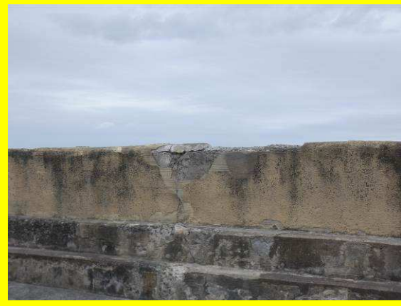
Continued spalling of repairs (/2201/C11)
