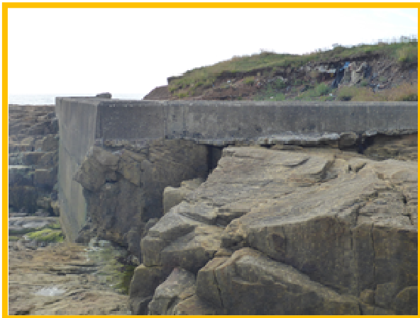
Seawall with undermining and outflanking (/3501C08)
