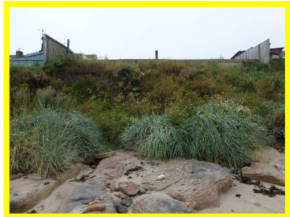
Retreat of slope, risk of out-flanking adjacent defences. (/1701C24)
