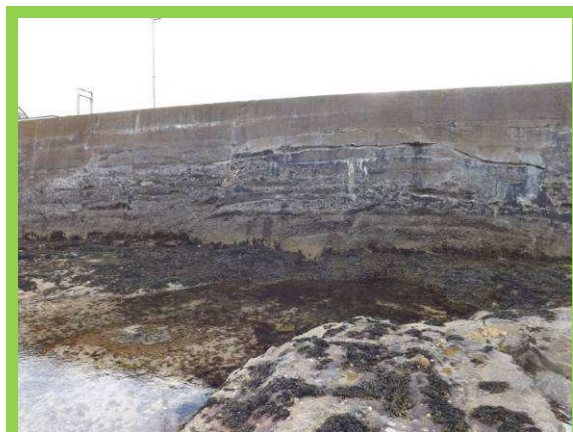
Old crack not noticeably worse 1701/C07
