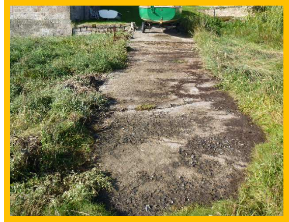
1401/ C23, Slipway in poor condition.
