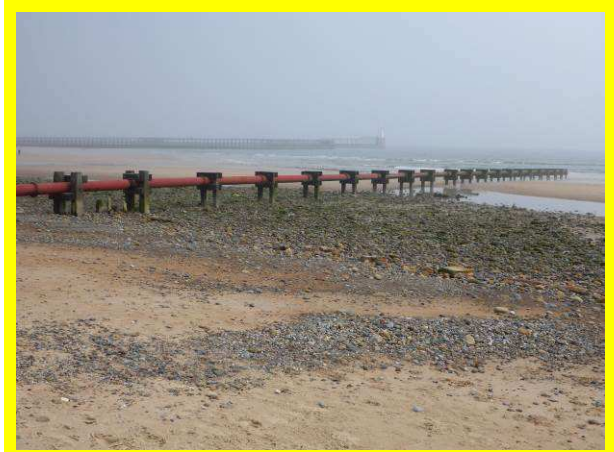
Cobble lag on mid beach by outfall (/4201C11)
