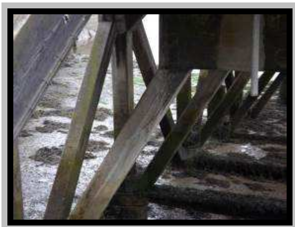
901c07 - 2016 spalling and repairs to RNLI .
