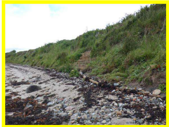
Local defence at toe of eroding cliffs (/2601C08)
