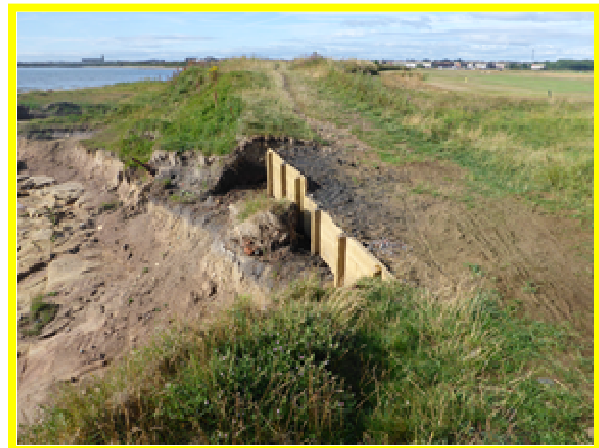
Eroding cliffs/dunes at Newbiggin Moor golf course (/3501C04)
