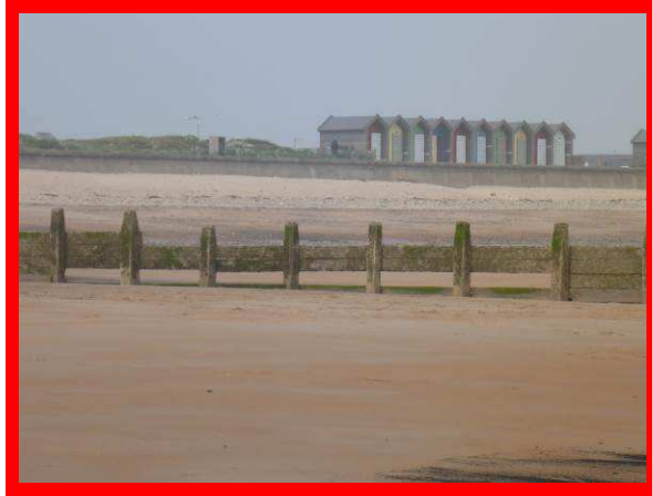
Missing boards from northern groyne (/4301C01)
