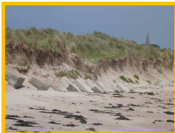
Eroding dunes at northern end of Birling Carrs frontage (/2901C01)
