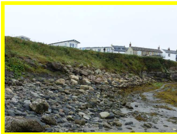
1701/C19 minor erosion above rock
