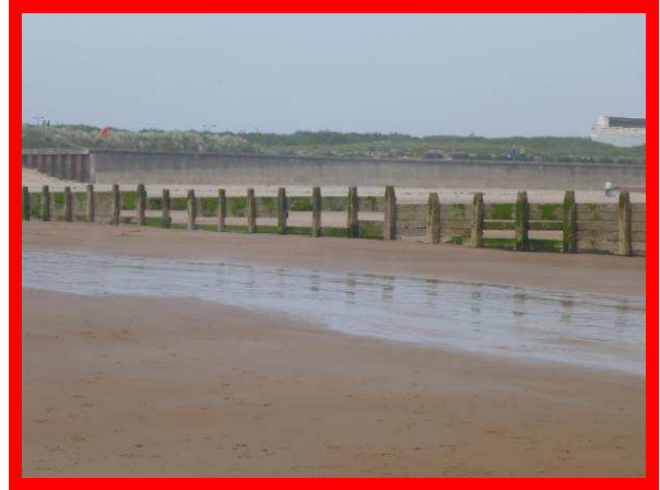
Missing boards from central groyne (/4301C01)
