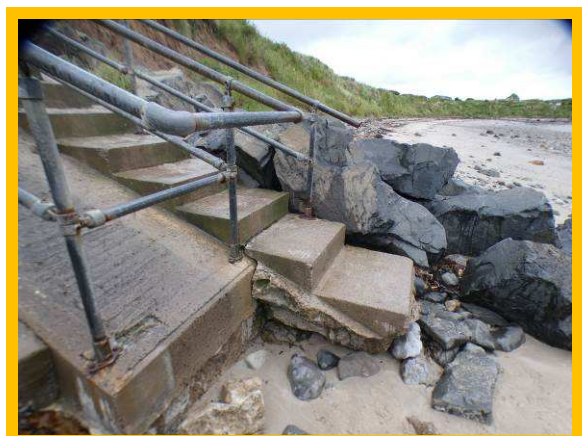
Lower beach levels exposing additional toe. (/2601C09)
