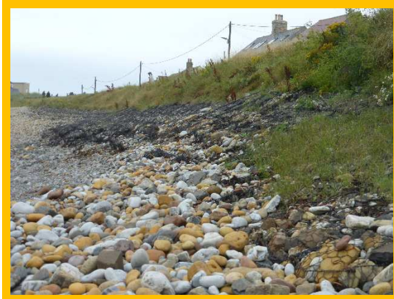
Failing mattresses at Beadnell North (Lady's Hole) (/1701C39)
