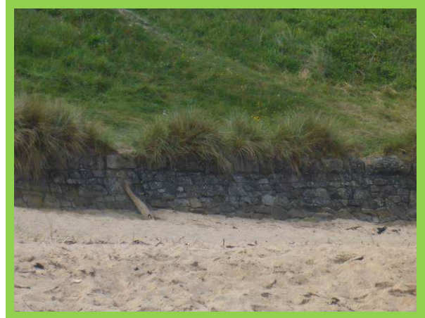
Stable dunes and good condition low wall at Sandy Island (/4401C01)
