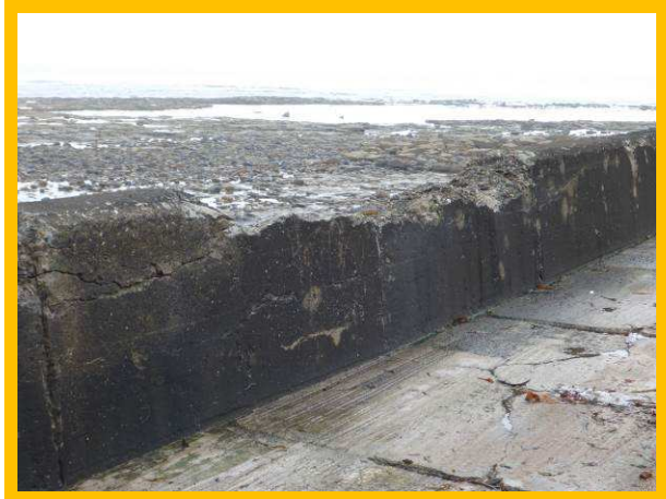
Damaged wall crest to landward section of Blyth East Pier (4001C04)
