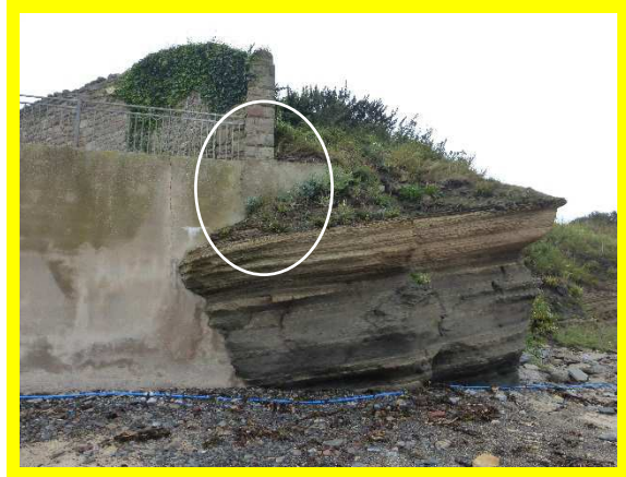
Cracking of seawall at transition with undefended frontage (/1701C31)
