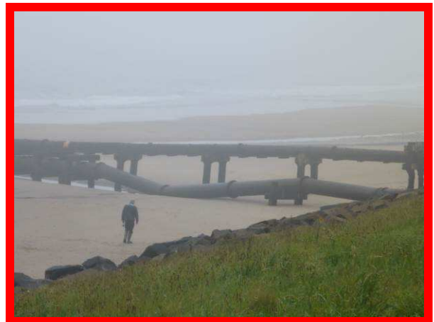
Failed section of outfall pipe (/3901C05)
