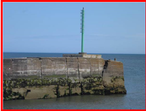
Seaward end of North Pier in very poor condition (/3001C02)
