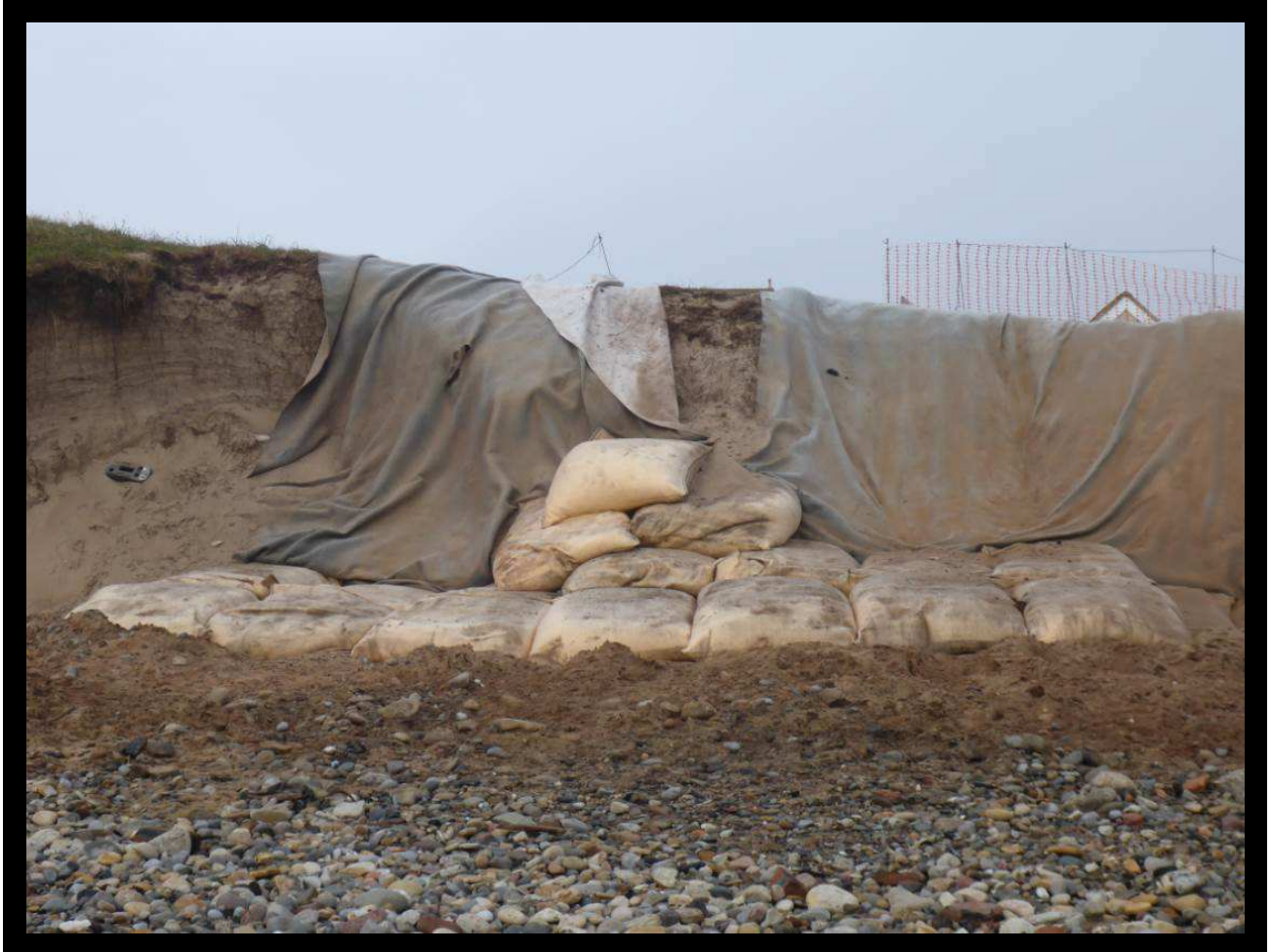
Dune stabilisation works at landfall of Blyth Offshore Demonstrator Windfarm export cable (/3901C04)
