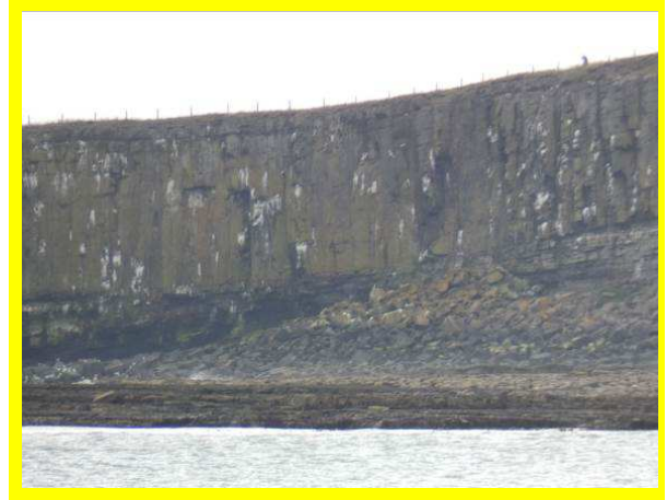
Localised rock fall at Castle Point (/2001C05) 2018
