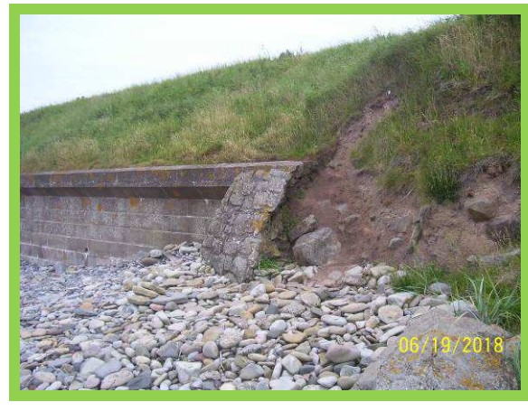
Outflanking of northern end of wall 1701/C54 - 2018
