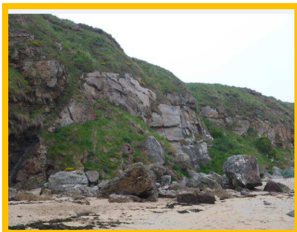
Past rock fall in cliffs at Green's Haven (/0701C05)
