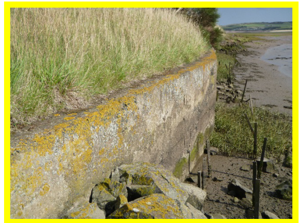
1401C14 – Concrete wall in fair condition. Timber toe erosion protection in poor condition.
