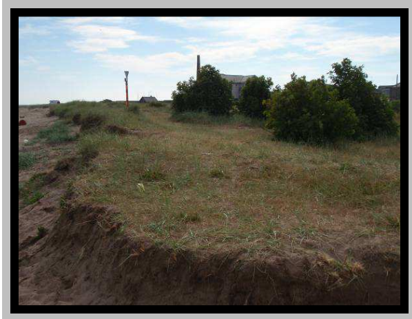
901c08 - erosion in 2012.
