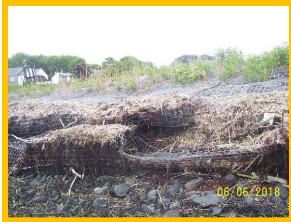
901c04 severe damage 2018.
