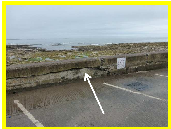
Old crack not noticeably worse 1701/C06
