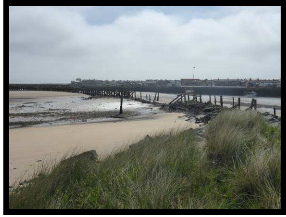
Dilapidated North Jetty (no asset reference)
