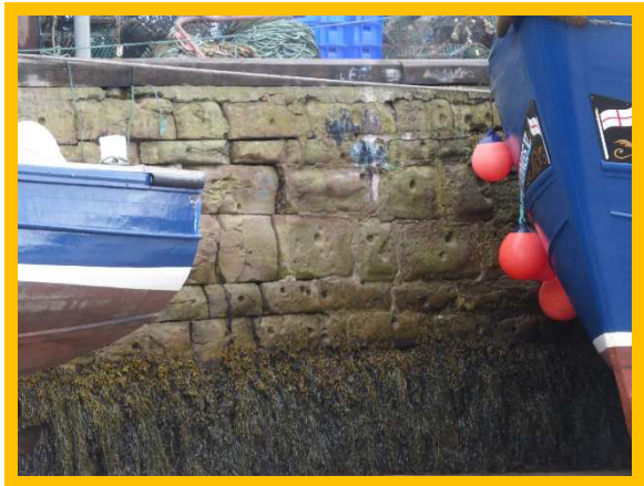
Full height cracking and loss of mortar to outer face 1701/C14
