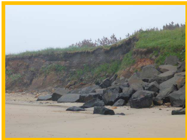
Erosion of cliffs at terminal end of rock revetment (/3901C03)
