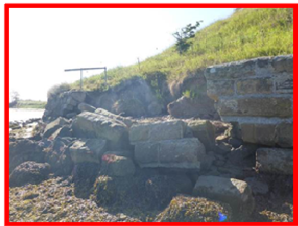
Defective section of masonry wall adjacent to collapsed section (/2801C13)
