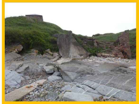
1101/c04 Outfall and concrete slope protection, cracked and weeping water 2018.
