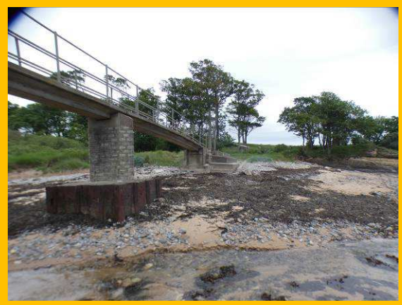
Detached toe beam at northern bridge abutment (/2501C01). Low beach levels
