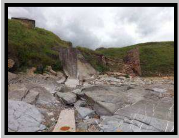
1101/c04 Outfall and concrete slope protection, cracked and weeping water 2016.
